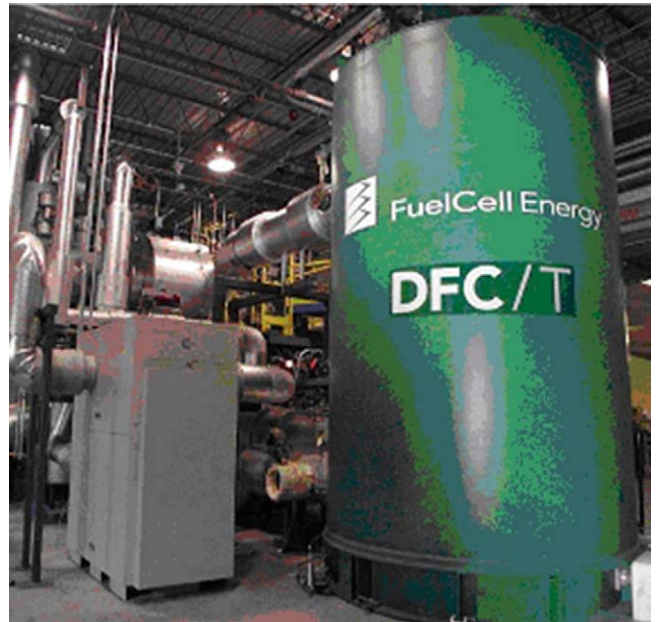
Fig. 4. A 250 kW DFC/T ® power plant in operation at FCE's headquarters, Danbury, CT.
