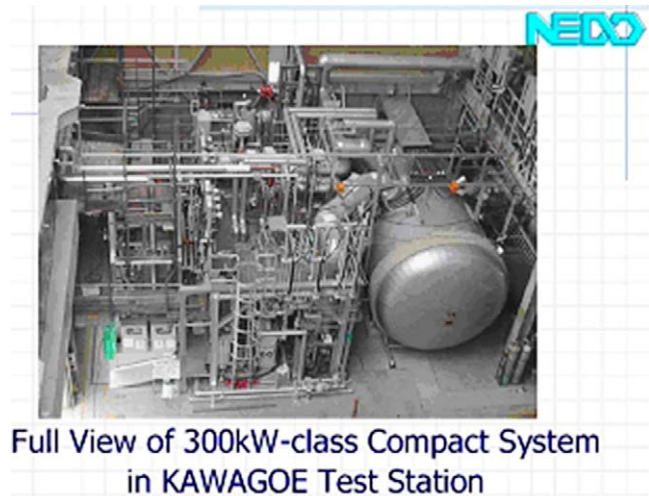
Fig. 1. A 300 kW compact system in Kawagoe.
